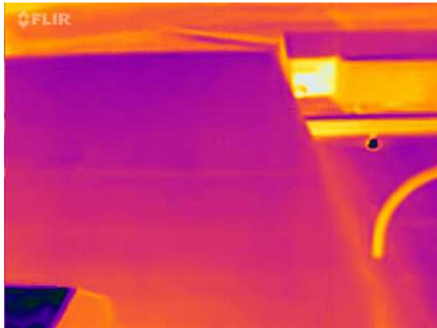
Flir One Photo standing on section A looking west, no anomalies found.
