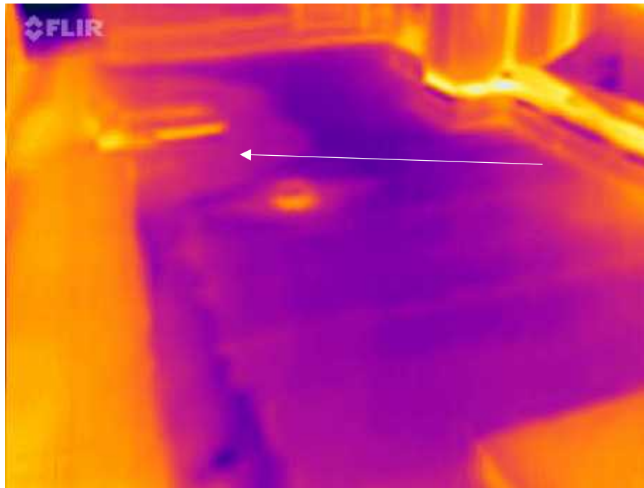
Flir One Photo looking north inside section H, due to the in closed space and the heat from the RTU thermal imaging was relatively difficult but one area was found to be suspected wet.
